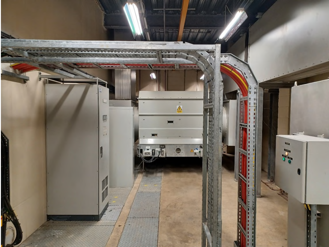
Figure 5 - View Inside R1 GCB Area
